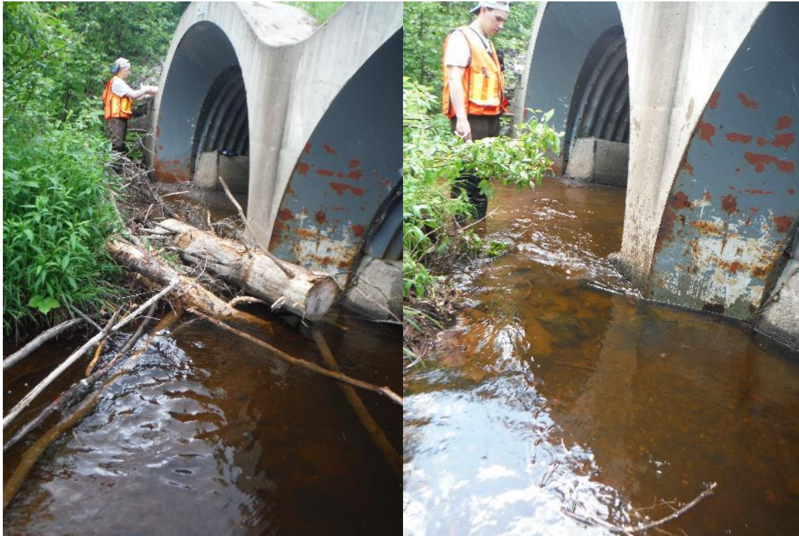
FIGURE 4. A DEBRIS BLOCKAGE BETWEEN CULVERTS 2 AND 3 AT A CULVERT ON MANZER BROOK WAS REMOVED, WHICH IMPROVED THE FLOW OF WATER. CULVERT 1 HAD A LARGE TREE INSIDE OF IT THAT COULD NOT BE REMOVED WITH THE EQUIPMENT WE HAD.
