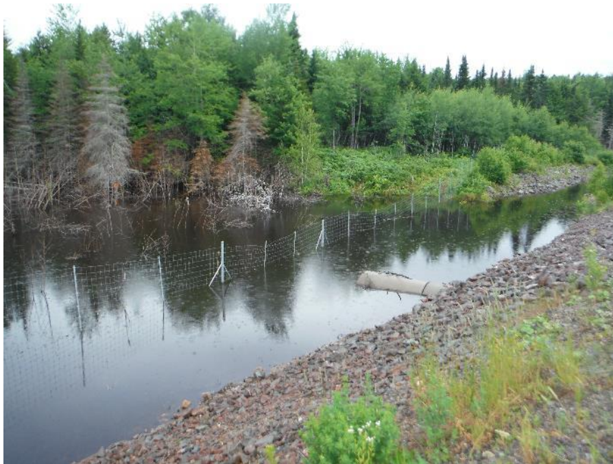
FIGURE 3. BEAVERS HAVE FLOODED THE UPSTREAM PORTION OF THIS SMALL STREAM BY BLOCKING THE INLET OF THE CULVERT.
