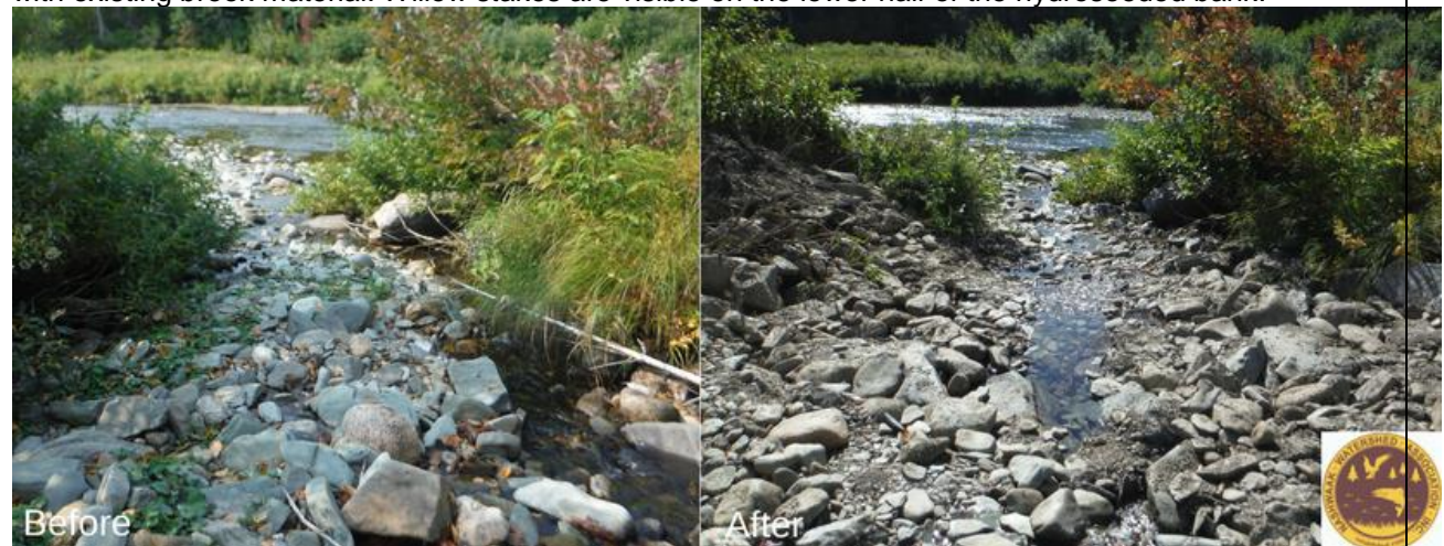
Looking downstream at the mouth of MacPherson Brook before (left) the rock weir was installed, a gravel island had built up and was channeling water to either side, which was causing more bank erosion. After (right) the installation of the sunken rock weir, water has been channelized into the middle, which will also improve fish passage at low flow conditions.
