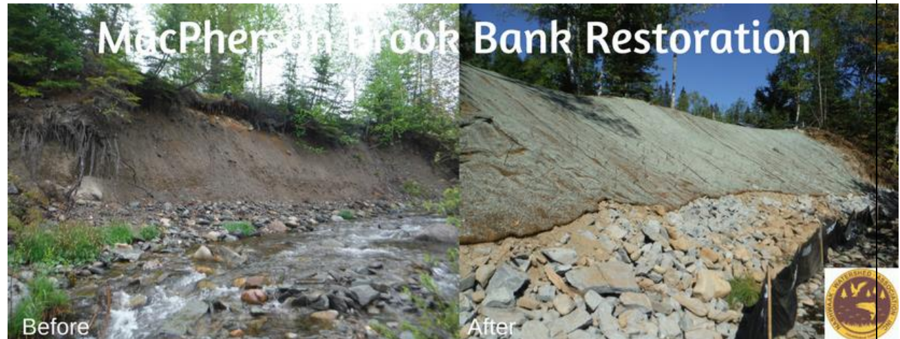
Previously (left), the bank was almost vertical and overhanging in places. After (right) the bank had been resloped to 1.5:1 and wrapped with erosion control blankets. The rock toe is made of R50 riprap mixed with existing brook material. Willow stakes are visible on the lower half of the hydroseeded bank.
