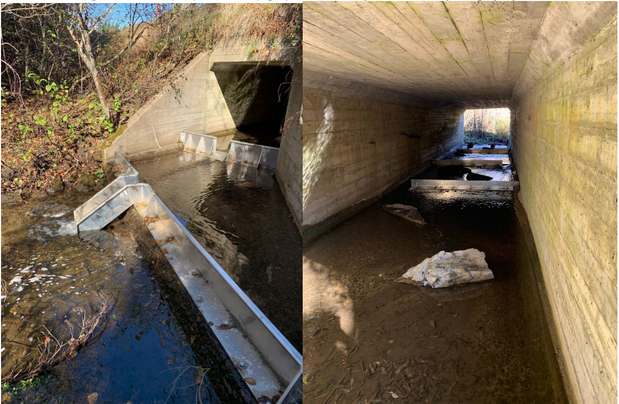
Figure 5. Details of the East Ryan Brook fish passage project showing the chute and first two baffles (left) and the upper three partial baffles (right) as well as the large rocks placed to provide microhabitat in the pipe.
