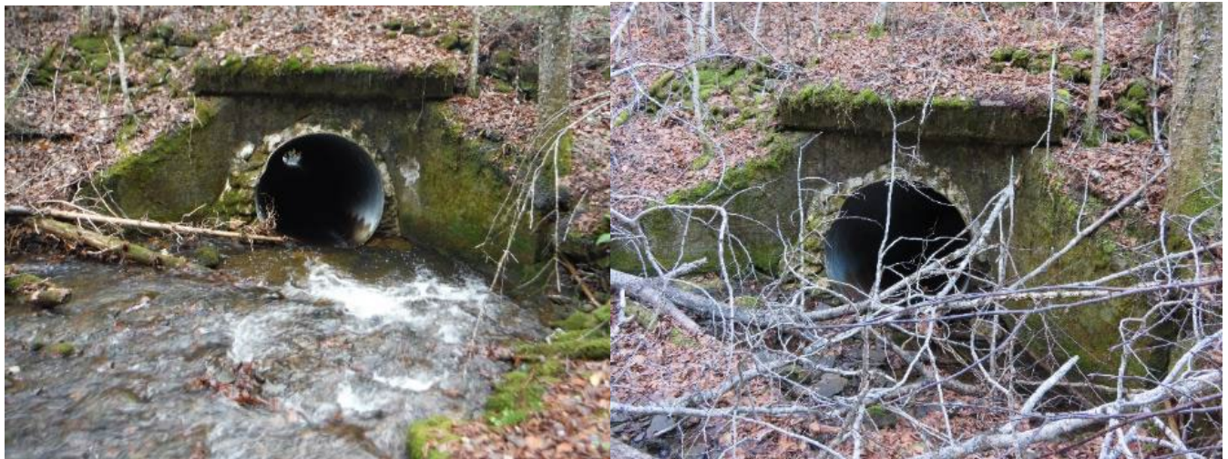
Figure 13. The inlet of the Porters Brook culvert in 2017 (L) and in 2020 (R). Many large trees have fallen in the stream and debris has started to clog the stream just above the inlet.
