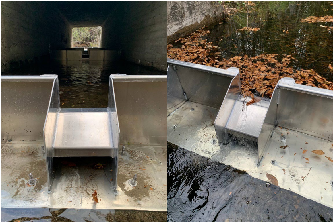
Figure 8. A close-up shot showing the weirs installed for the Limekiln Brook fish passage project in 2020. The weirs were not fully installed at this point, so water was just starting to flow over the chute.
