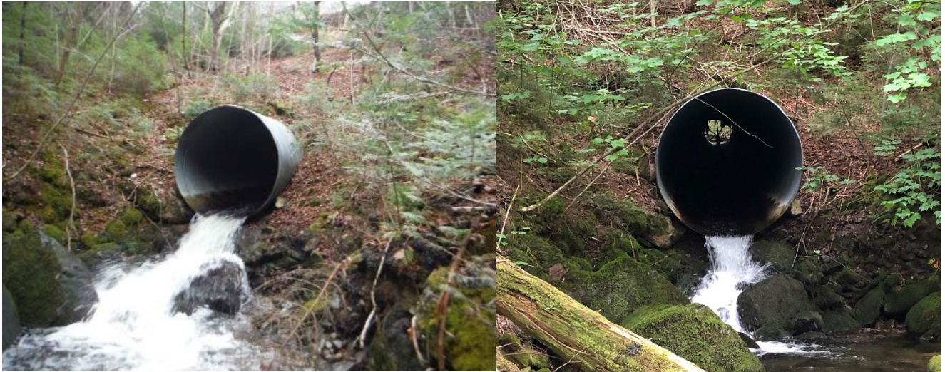
Figure 12. The outlet of the Porters Brook culvert in high water conditions in 2017 (L) and in low water conditions in 2023 (R).
