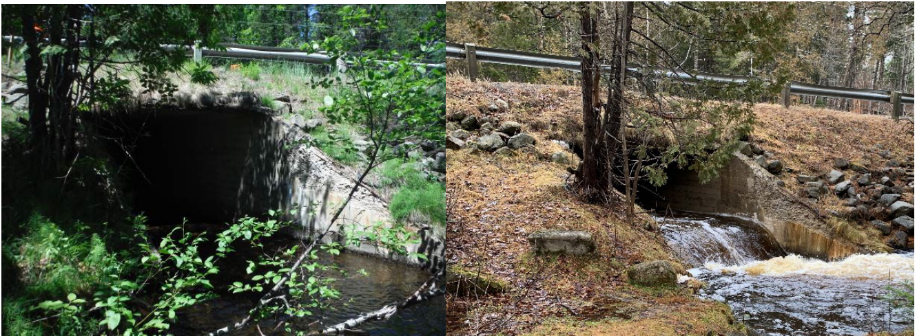
Figure 7. Road-stream crossing at Limekiln Brook in 2020 (left) before remediation and in 2023 (right) during high-flow after structure was installed in 2020.
