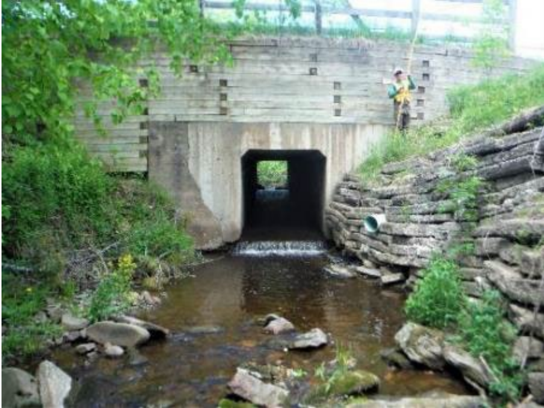
Figure 9. Picture looking upstream in McConaghy brook (MC01). This site is a full barrier to fish passage, blocking 4.2 km 2 of viable upstream habitat.
